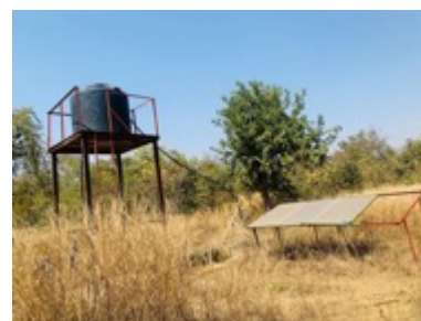
1000-liter water tank and 3 school panels with metal brackets
